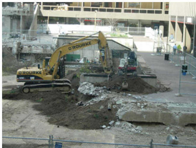
Work began to clear the planting beds along the Fifth Third Tower
