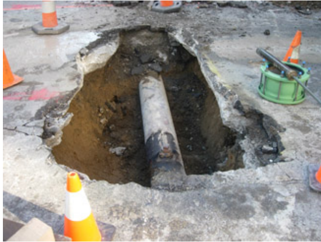
Underground pipes exposed in order to be shutoff during demolition Photos from previous updates
