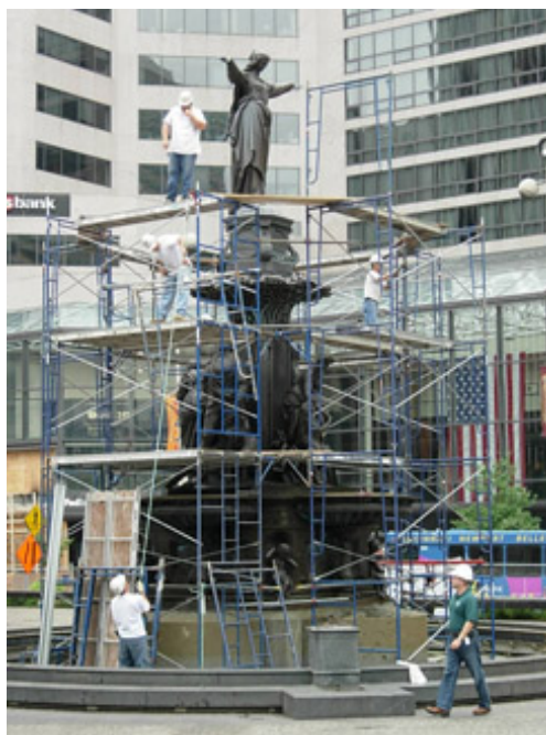
Scaffolding is constructed around the Tyler Davidson Fountain to allow for its safe removal from the Square
