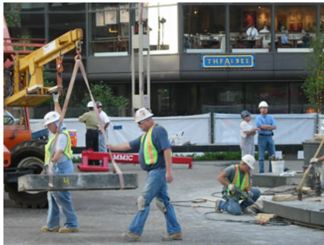
Construction workers remove the granite donor ring surrounding the Fountain in order to safely store it until it rejoins the Fountain in the revitalized Square
